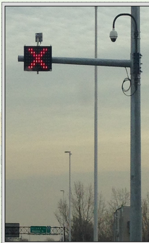
The Lane Control System on the NBHCE, which lets drivers know when the shoulder is open to traffic, will be decommissioned starting on or about May 6, 2019.
